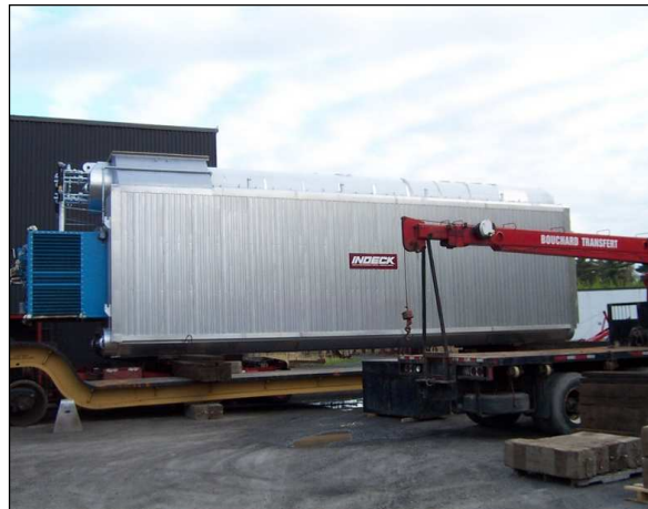
Boiler of 110 tons
